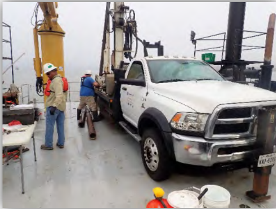
1. Truck-mounted drill rig in braked position on work deck of Spud Barge.
